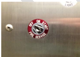
Figure 2. Fire Service Control Switch (three position)
